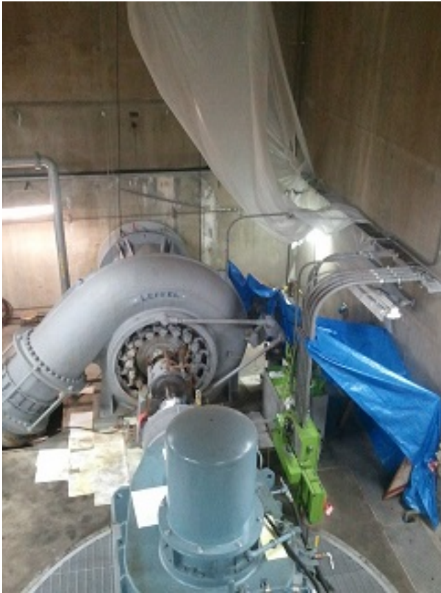
Image 1. Tarps covering equipment in SFL AWS turbine room.
